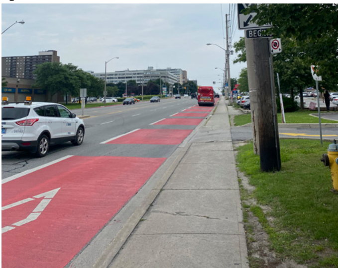
Figure 5.1: Narrow Sidewalk Abutting Fast-Moving Traffic, Eglinton Avenue East near Markham Road
